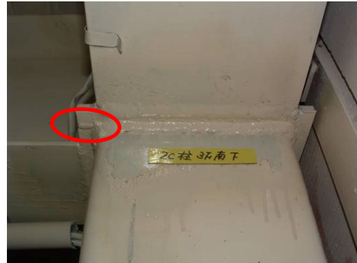
2 C柱 3階 南西面 下側
